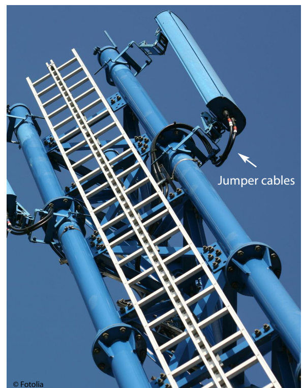
GSM Base station
